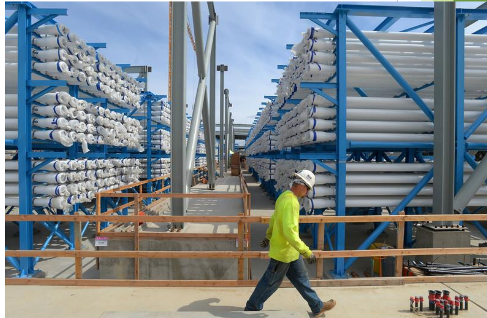
Carlsbad Desalination Plant, 2014
